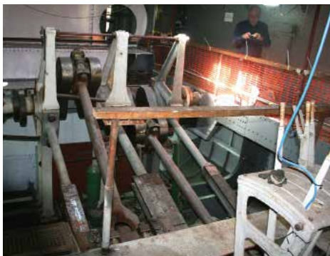
The Medway Queen's engines; fitted but now awaiting a boiler – and a clean up.
