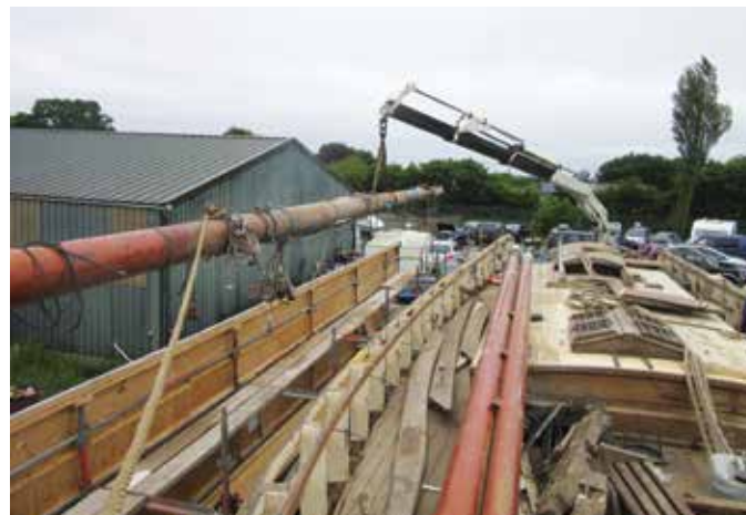
Moving spars off the deck before putting a roof on the shed.
