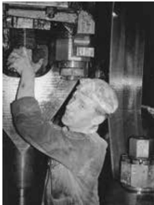
The engineer is removing the piston rod nut to take out the main piston.
