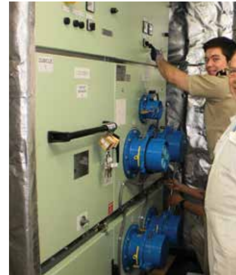
Shore power connection.
