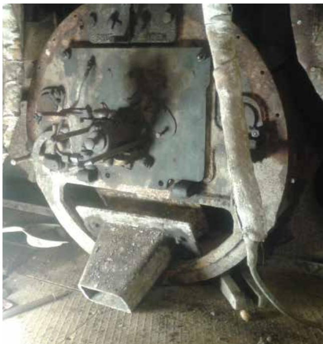
Bottom (ash) door removed from its hinges to reduce weight of the frontage.
