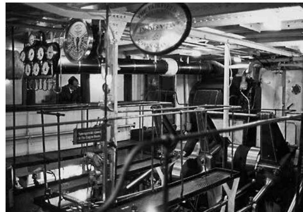
Britannia's engine room.
