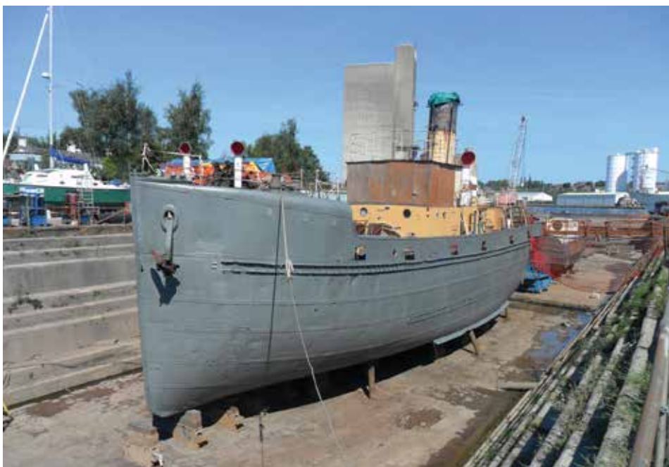
Plating has been completed and the undercoat has been applied to the hull.
