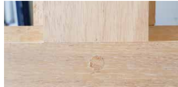
Close up detail of the pegged mortice and tenon joints between the stiles and rails.
