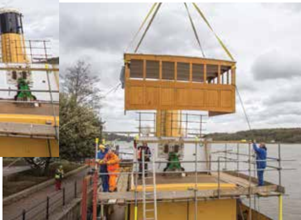
BELOW: On its final approach – the wheelhouse is gently lowered into position to begin a new era in the ship's future.
