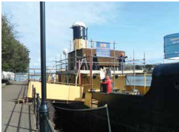
Removing the old plywood cladding from the wheelhouse in preparation for the new one's arrival.
