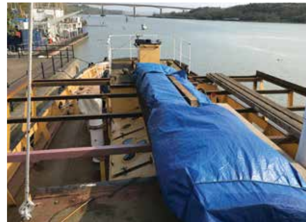
LEFT: The next big job after the wheelhouse is the rebuilding of the boatdeck. With new steelwork in place, the timber, under the tarpaulins, is ready to be fitted.
