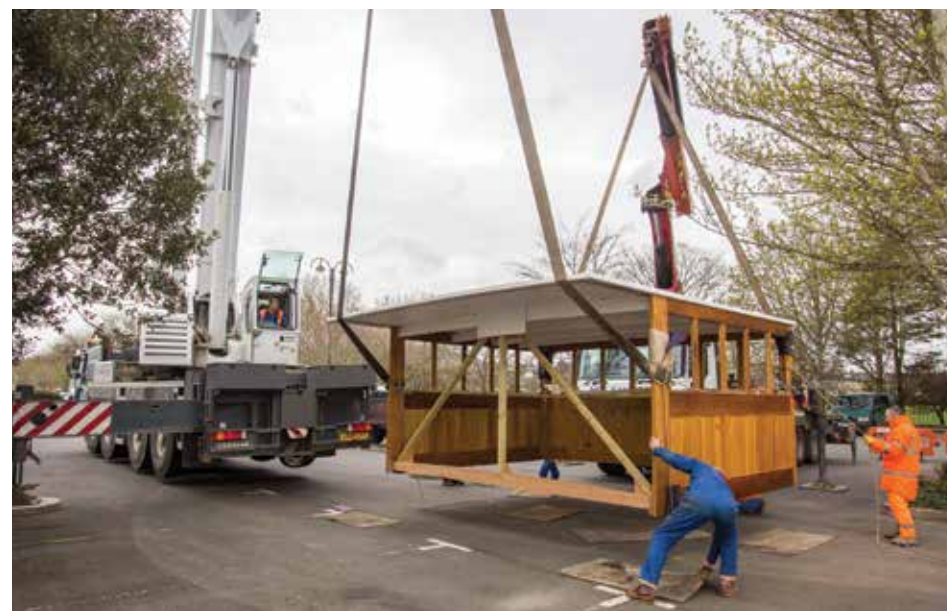
Landing the new wheelhouse in the car park, having turned it upright.
