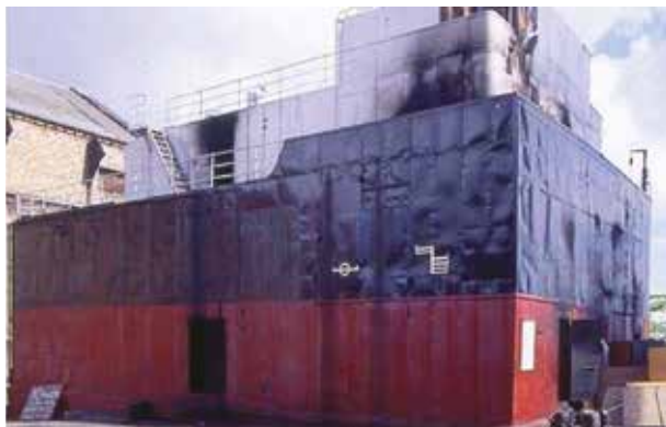
McDonald Road fire fighting facility looking a bit scorched.
