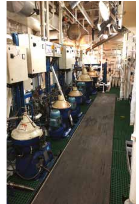
The Purifier Room.
