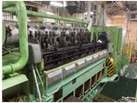
Generator after overhaul.
