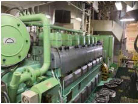
Generator before overhaul.
