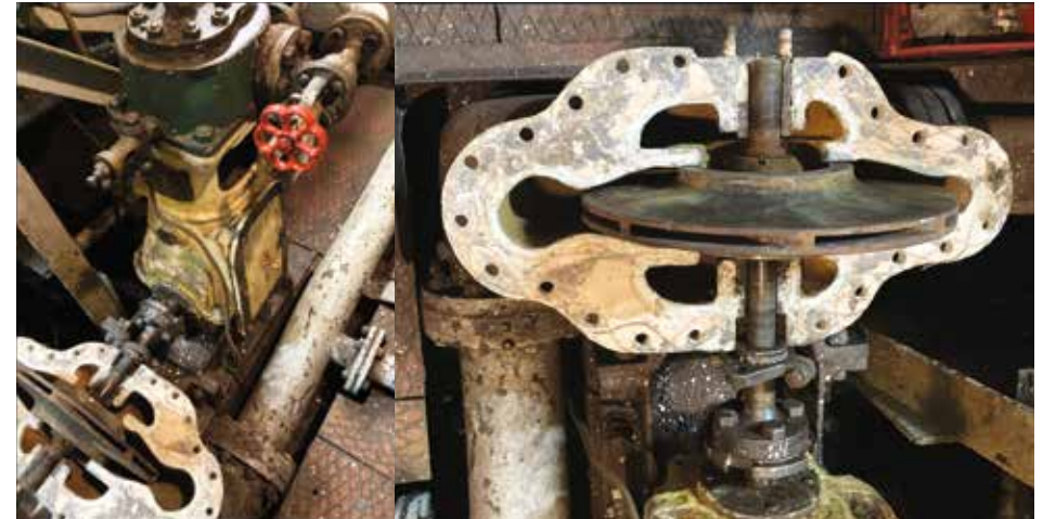
This pump is driven by a single cylinder reciprocating steam engine.
