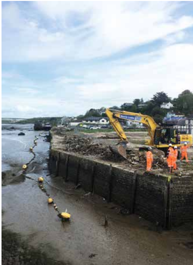
Repairs to sea wall at East-the-Water in May 2023. This section of wall originally was constructed in 1887 after the closure of the last shipyard. Courtesy Mike Teare
