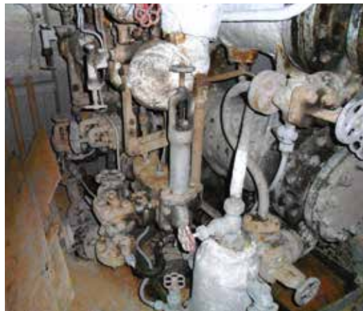
The Wallsend Howden fuel system before...
