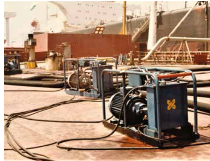
Hydraulic power packs driving the pumps.
